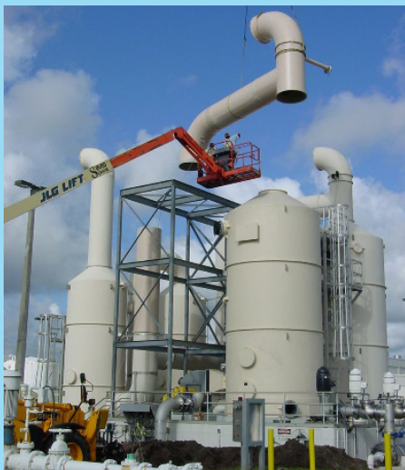
Figure 9: Addition of Second Degasifier Tower
