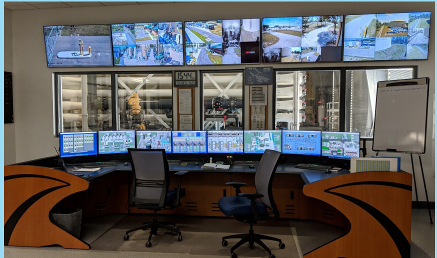
Control Room Monitoring Data
