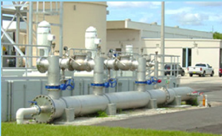
Figure 6: Degasifier Clearwell with Transfer Pumps
