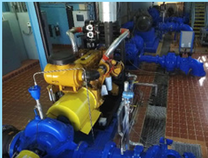
Figure 10: High Service Pump Room with Diesel/Electric Pump (HSP-1)
