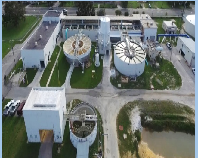
Figure 2: Membrane Building (Upper Left), Lime Softening Units/Filters (Right), and Lime Sludge Thickener (Lower Left)
