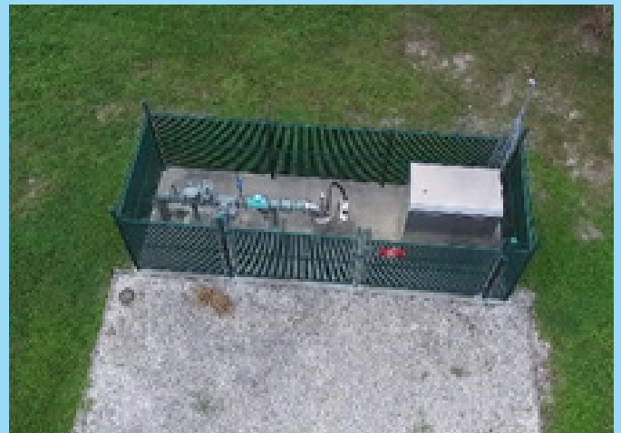
Figure 7: Off Site Surficial Aquifer Well
