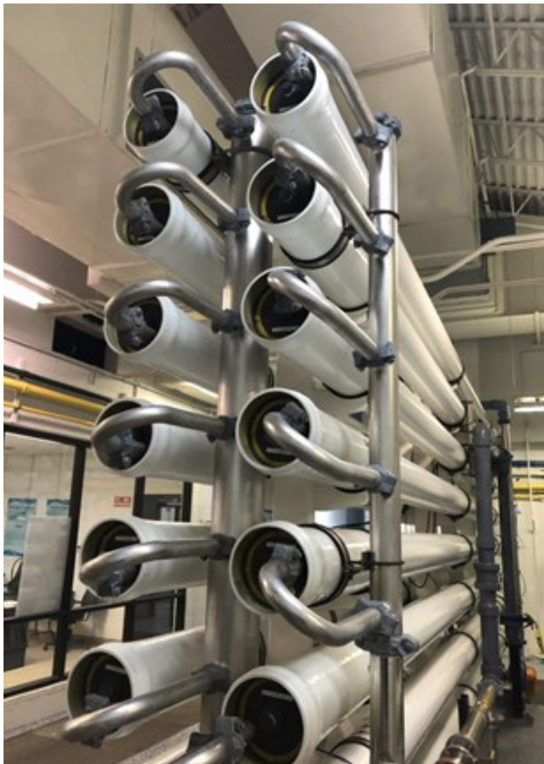
Figure 1. Example RO Train at Mount Pleasant Waterworks WTP #3
